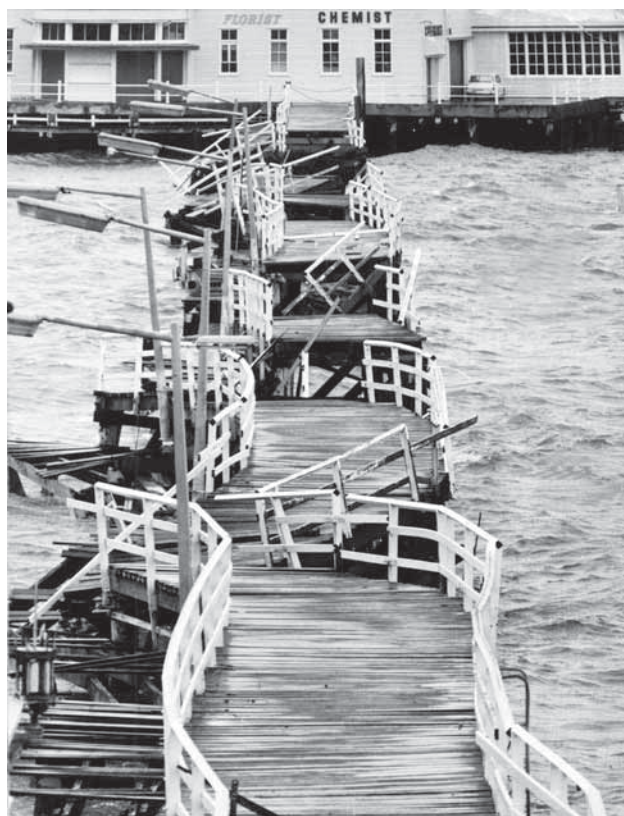
Storm damage to Manly promenade, Sydney 1974.
